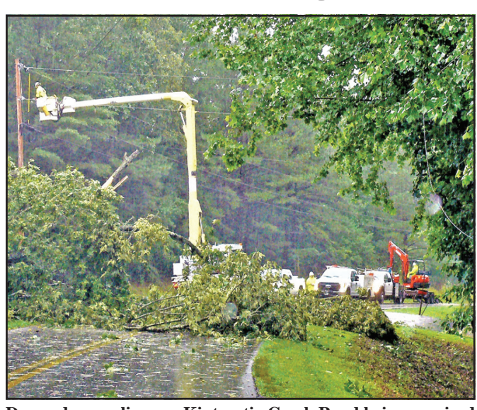
Downed powerlines on Kiutuestia Creek Road being repaired by Blue Ridge Mountain EMC linemen following an afternoon storm on Wednesday, June 27. Photo by Frank Uhle
